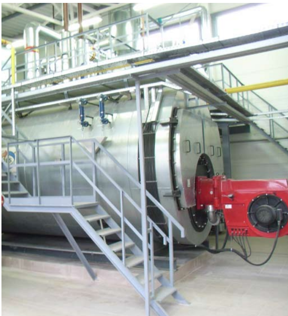
New high efficiency steam boiler at ScanDye which ensures optimal energy use.
